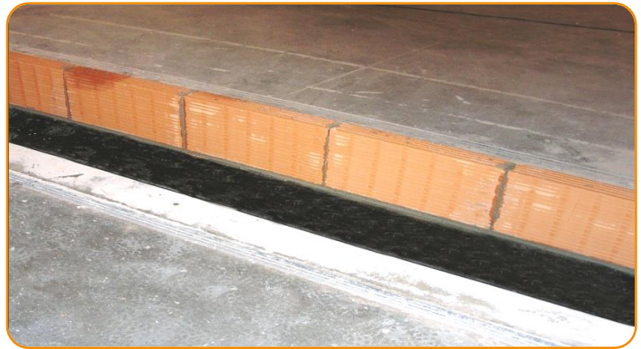
Over the Stywall, lay down a plaster bed in order to start to built up the wall
