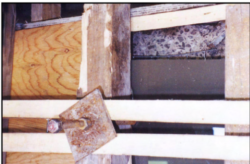
Autoroute 540/40, Quebec City, Quebec, Canada. Repair of pier cap as seen through Plexiglas formwork. No internal vibration was applied. AMBEX SCC flowed freely by gravity 11m (35 feet) into formwork.
