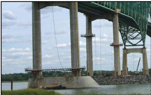
Laviolette Bridge, Trois Rivières, Quebec, Canada. 10,000+ bags of SCC were used to repair patches on bridge piers that were up to 60m (200 feet) high.
